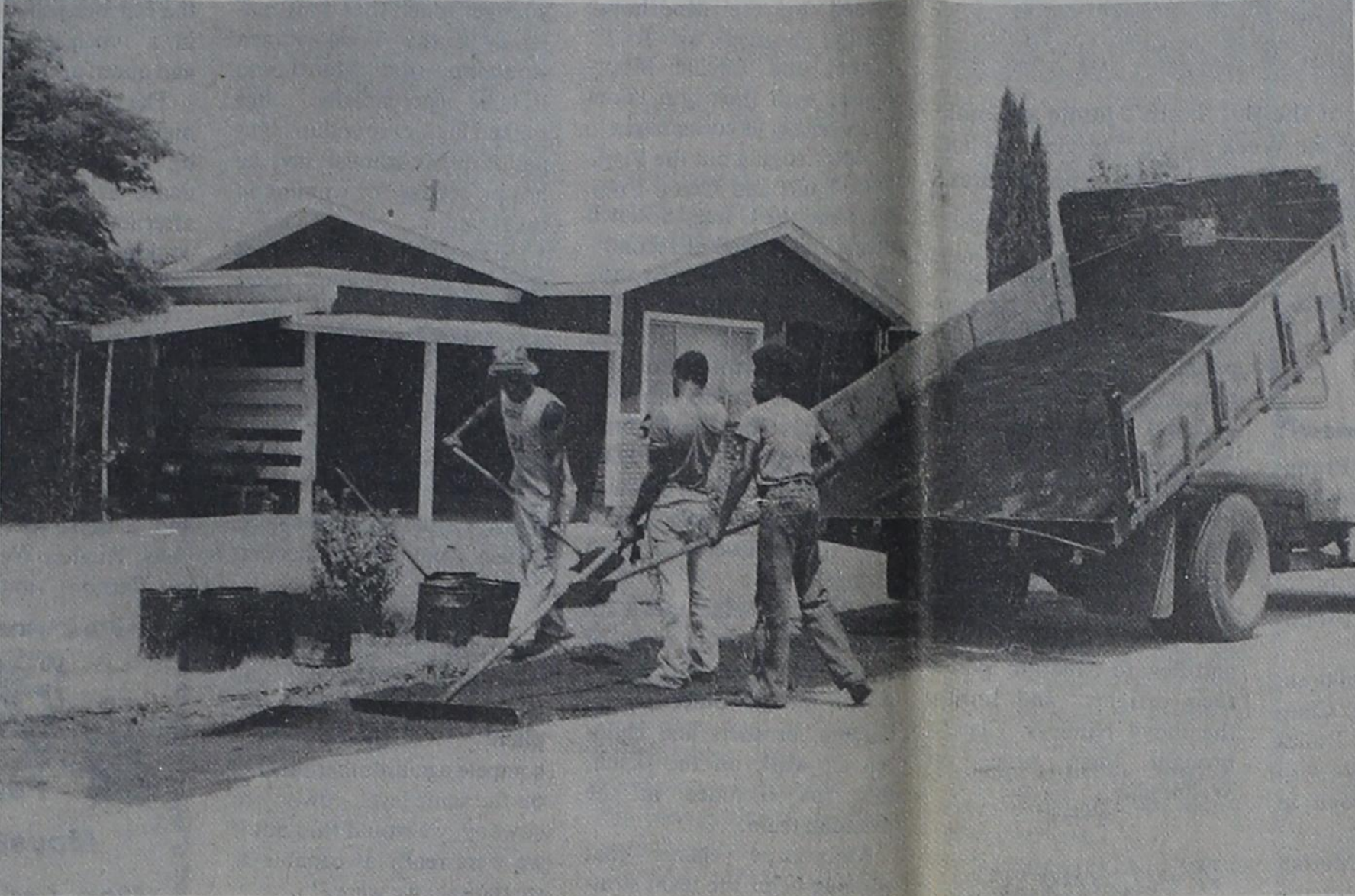
STREET REPAIRS: Work crew of the City of Munday are making repairs on Irving Street, getting it ready for a seal coat job. Workers have been busy repairing a number of the city's streets during the past several weeks.
