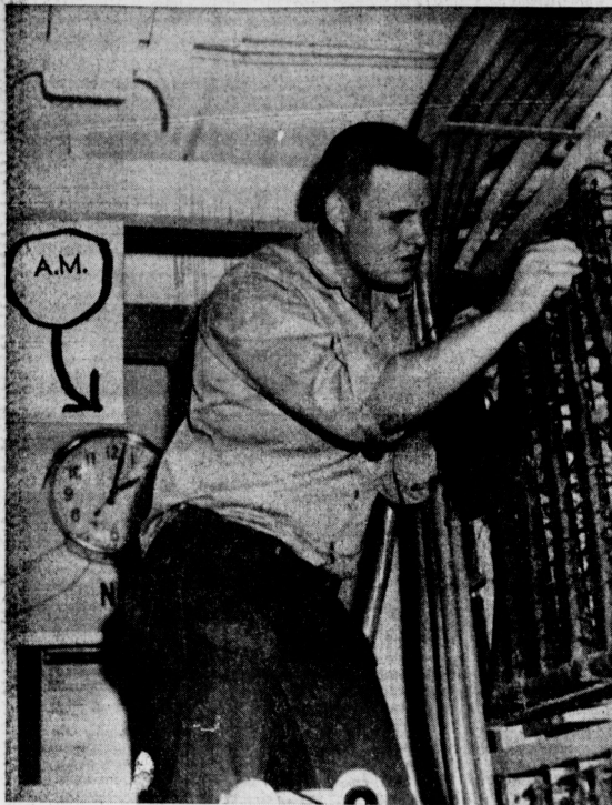
NIGHT CUT-OVER — Workmen these nights are cutting over a lot of numbers at the Muleshoe telephone office, making ready for General's big switch-over Aug. 15 when the system goes to a seven-digit system. The cutovers are being made in the middle of the night in order not to interfere with service. This is Merlin Neal doing one of the many switching jobs. (Journal Photo)
