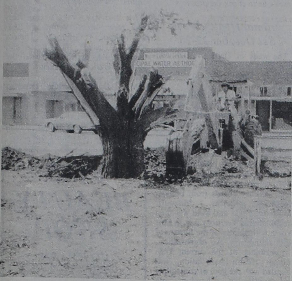
DESTRUCTION OF THIS LARGE shade tree is another reminder that progress is being made on the removal of the old city hall. This particular tree is being removed to make way for a parking lot which will be located adjacent to the new city hall building when it is completed.
