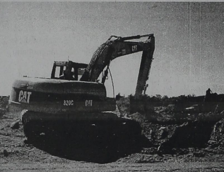
(HEAVY MACHINERY in T&P Industrial Park at site of Federal Express terminal under construction.)
