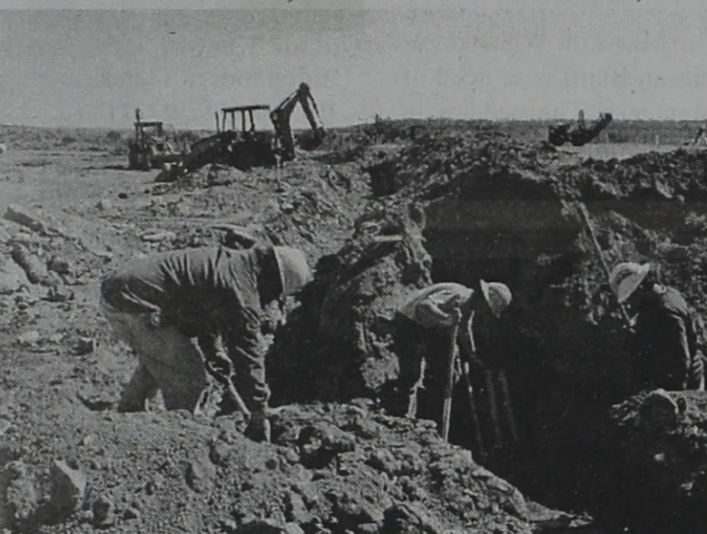
(This past week at Baird, Construction, workers pouring foundation for Baird's new Fed Express terminal.)
