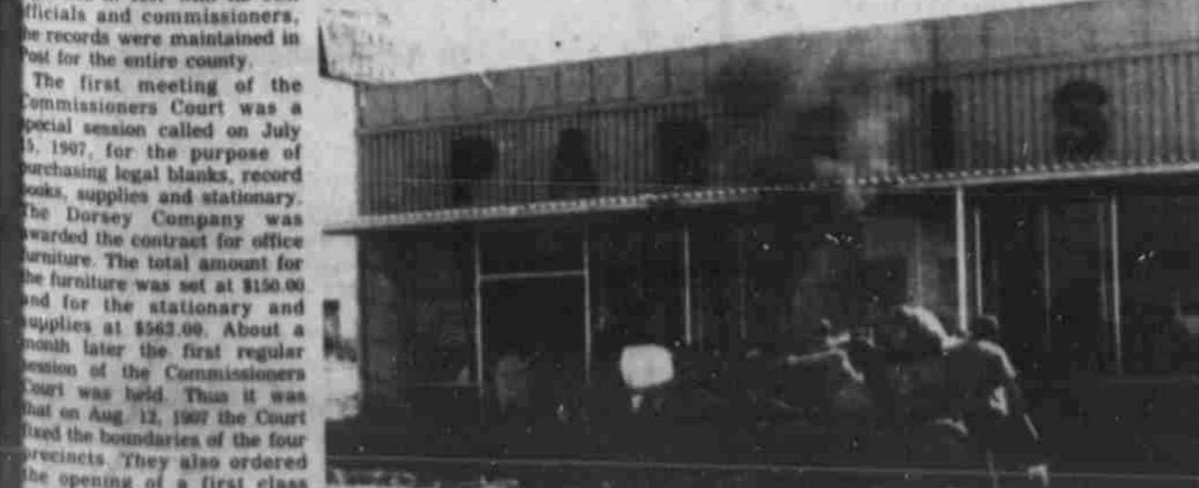
RENOVATION BEGUN — A bulldozer rips up parking area in front of the old Parrish Grocery & Market Tuesday as work begins on the remodeling of the super market building into the Post Community Center. Watching in foreground is Lubbock Contractor Lee Lewis who is in charge of the job.
