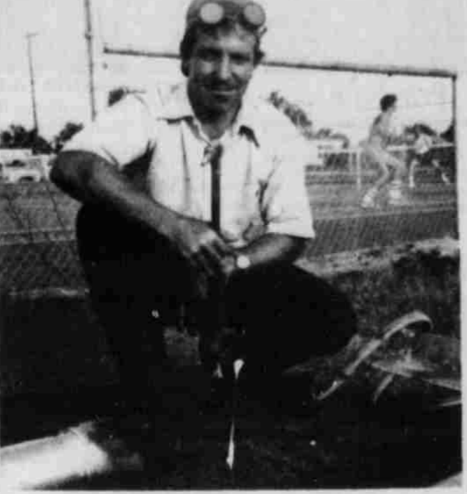
ERECTING TENNIS LIGHTS — Royce Hart and his blow torch are pictured above as he prepares to erect poles for lights at the local tennis courts. One light pole was erected Tuesday. According to Royce, tennis lights fund will be about $200 short and contributions can be made to the tennis lights account at the First National Bank.
