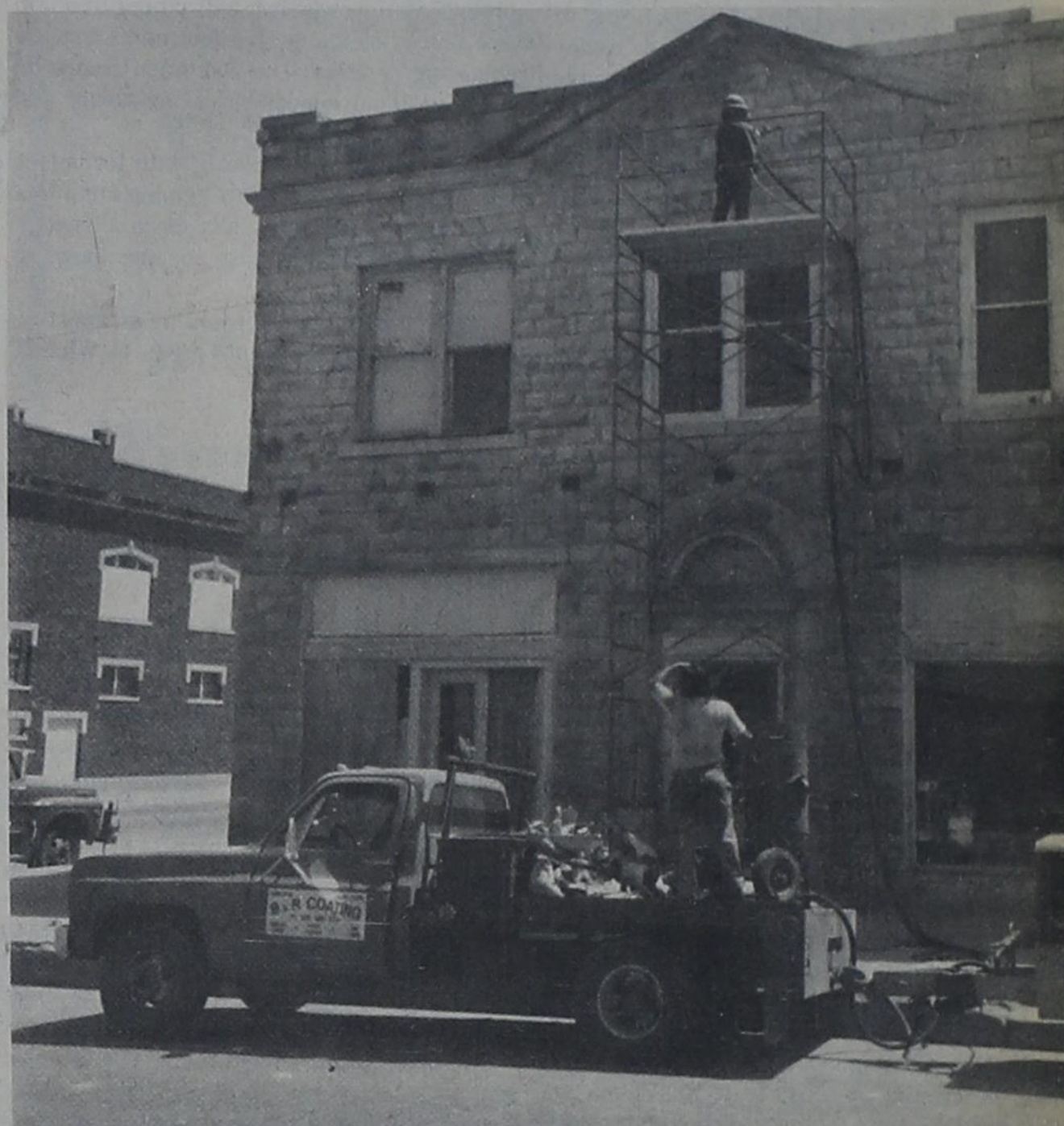
CLEANER FACE — Workers sandblasted the stone front of the historic Algerita Hotel last week as one of the first steps in the exterior renovation of the hotel by David Newby. John Bustos is at work high up on the platform while Johnny Garcia keeps the sand coming from the truck parked in the street below. — (Staff Photo)
