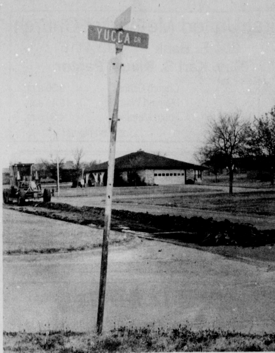
PROJECT UNDERWAY - City workers began tearing out the old asphalt on Wagonwheel from Johnson to Surrey Monday morning. The new surface is expected to be applied in about two weeks, after the base is compacted.
