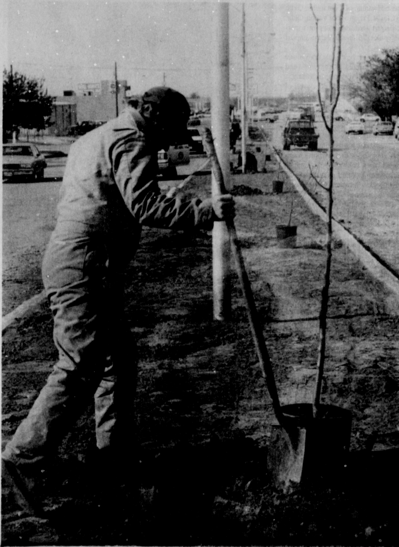
PARK AVENUE BEAUTIFICATION UNDERWAY - City workers this week began planting trees as part of the city's effort to improve the looks of the major thoroughfare. The rock covering has been removed and new soil filled in the median area of the 200 block. Work also commenced in the 300 block, and soon will start in the 100 block. Besides trees, ground covering grasses will be used, as well as garden areas, according to Sue Hatcher, who is coordinating the effort.
