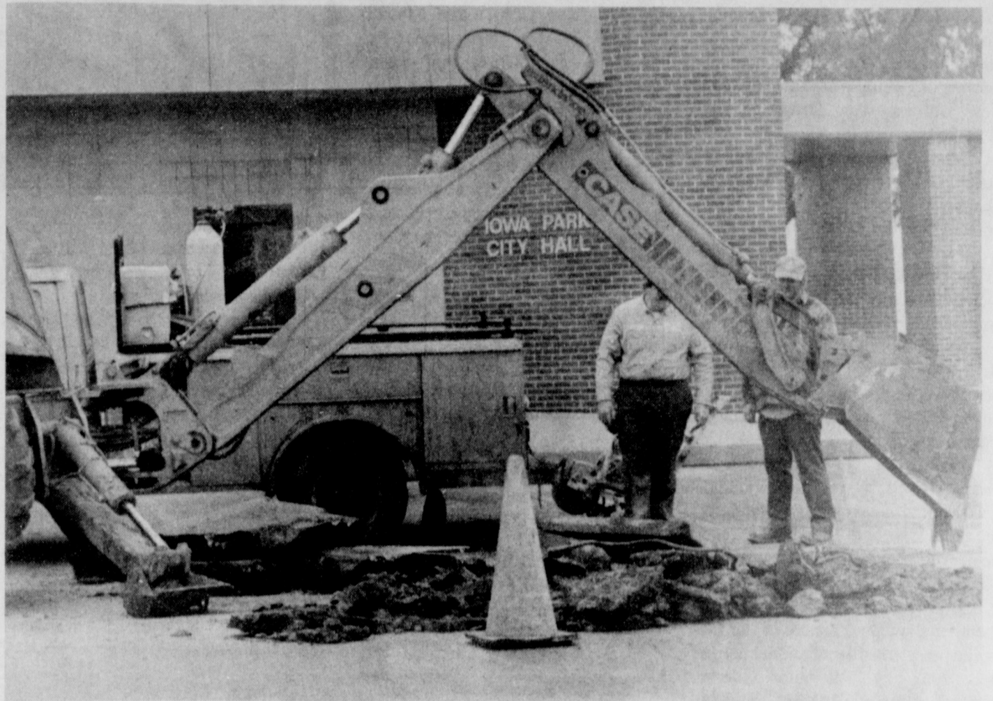
DIGGING FOR WATER - Iowa Park Water Department workers had to dig up a portion of Wall Monday, to repair a broken main that had been leaking more than two weeks. They had been forced to wait until they had caught up with numerous breaks in lines over the city, apparently caused by an extended dry period. Once they reached the break, they waited until after 10:30 p.m. to make the repair, because they had to shut off service in the north part of town to do it.
