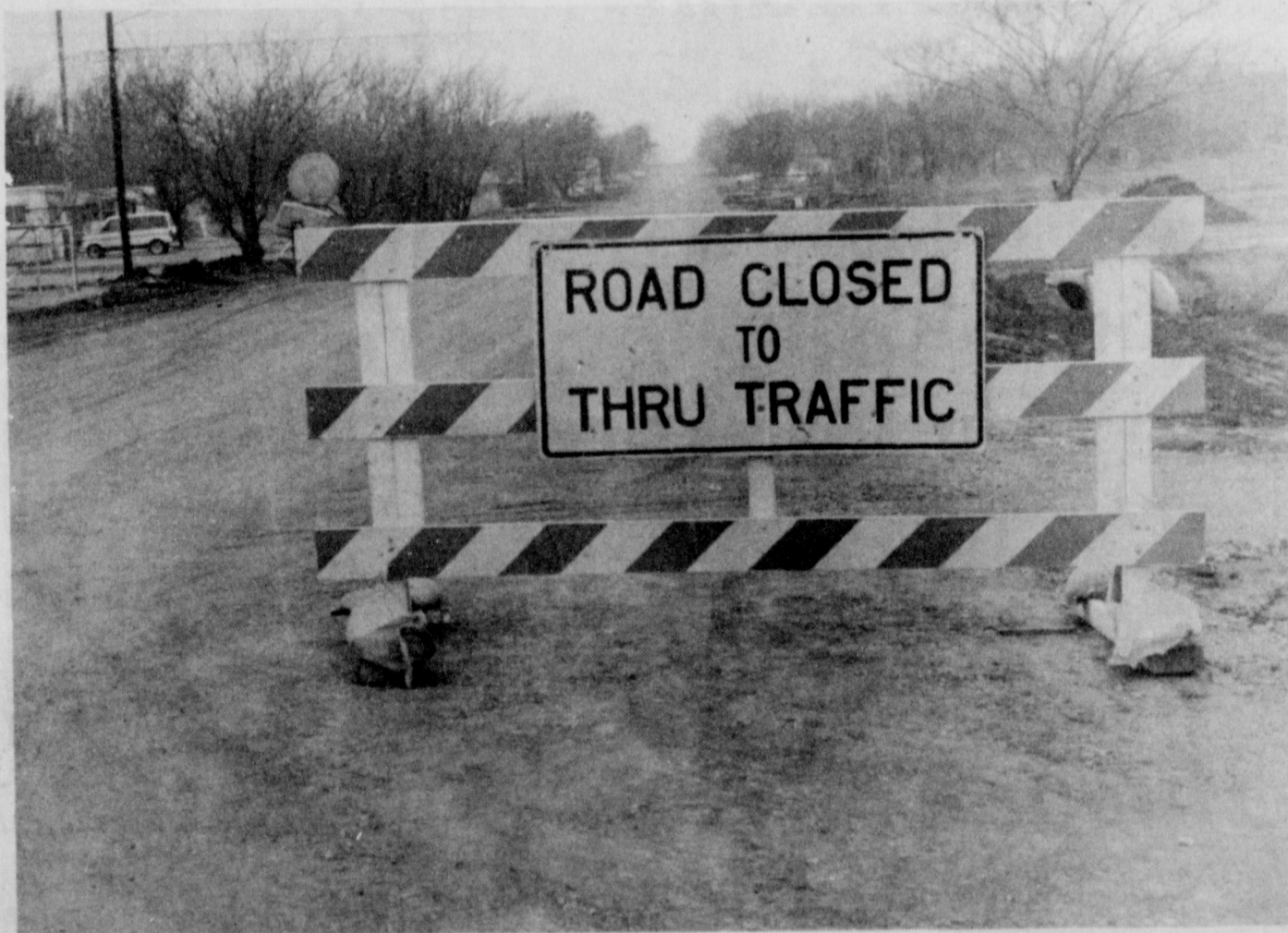
WASHINGTON STREET PROGRESS - Weather permitting, workers are to begin shooting the gravel base on Washington Street with a prime coat, as a prelude to laying on hot mix asphalt paving. Ray Self, engineer for the Department of Transportation, suggests that anyone having to drive on the prime coat, which can be "very black and sticky," to do so slowly, to prevent the substance from splashing on the vehicle. Once the prime is cured, Self said the asphalt paving will be applied.
