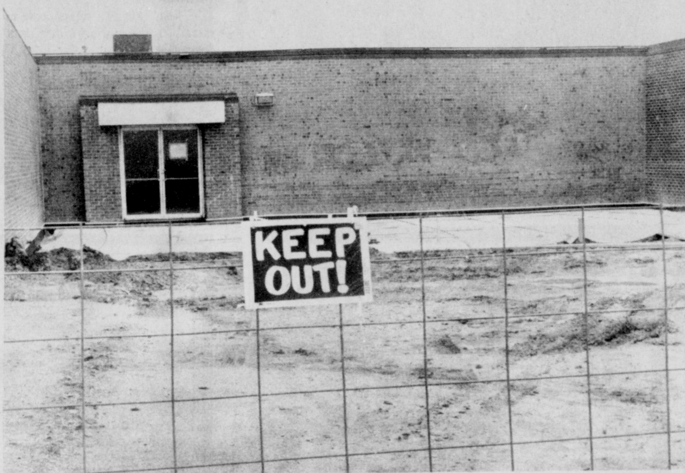
CONSTRUCTION UNDERWAY for the newest addition to Iowa Park High School was delayed Tuesday. Workers were scheduled to pour concrete, but that was postponed because of overnight rains. The addition will house a special education facility, and will cost approximately $90,000.
