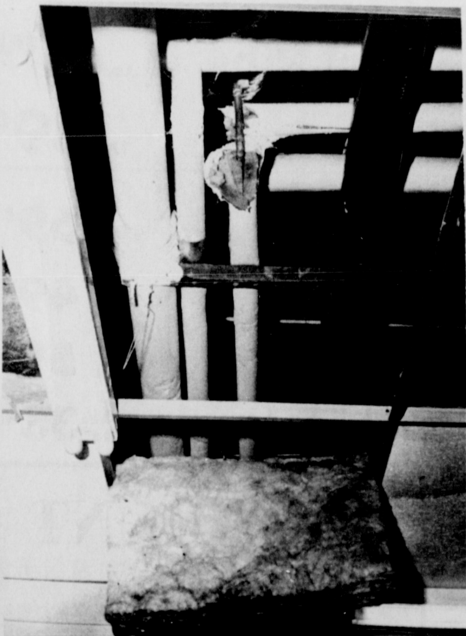
BURST WATER PIPE ...high school damage inflicted.
