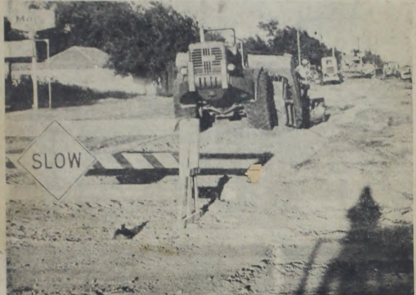
Could this be Main? — Yep, only a few days ago. All the loose dirt and construction as soon as the paving is completed to join the curbs.
