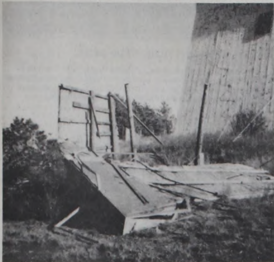
Wind storm damage at the old Mid-Way Theater between Turkey and Quitaque.
