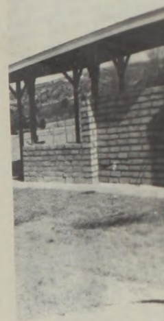
Brick windbreaks are being built at Lake Mackenzie this winter. Authority has also requested Texas Parks and Wildlife building two boat docks, also.
