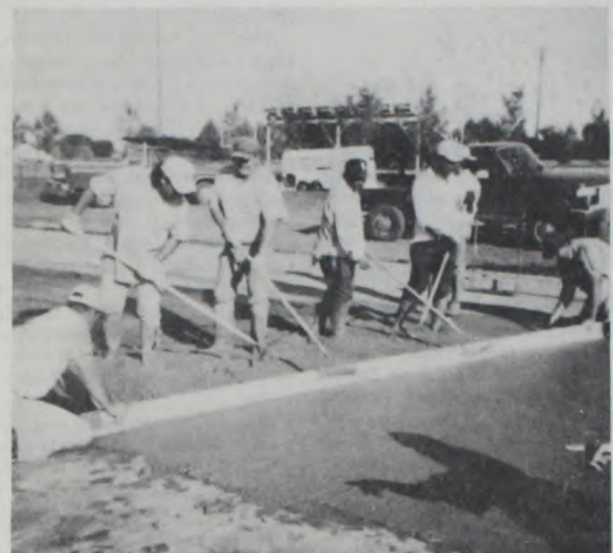
Volunteer workers smooth cement on the floor of the new Valley Agricultural class building. (Staff photo)
