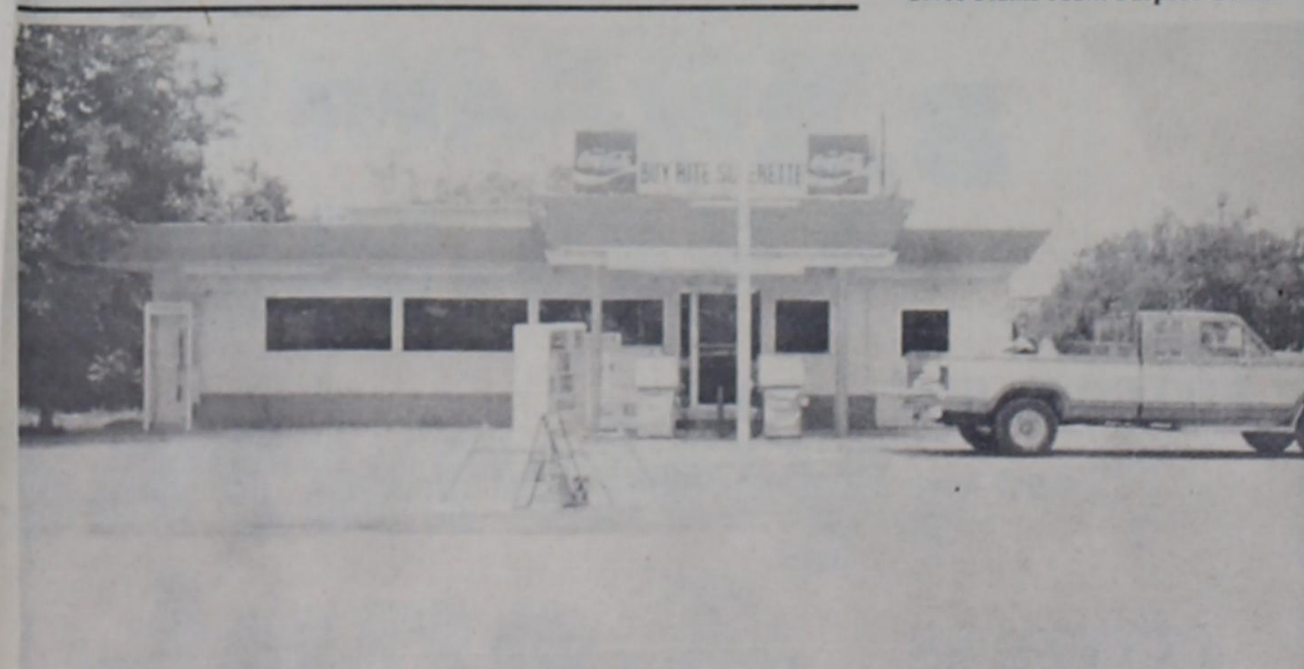
BUY-RITE REMODELING — Reed Superette is near completion. Mr. and Mrs. Bill Lewis ask that you watch for Construction announces that Buy-Rite
