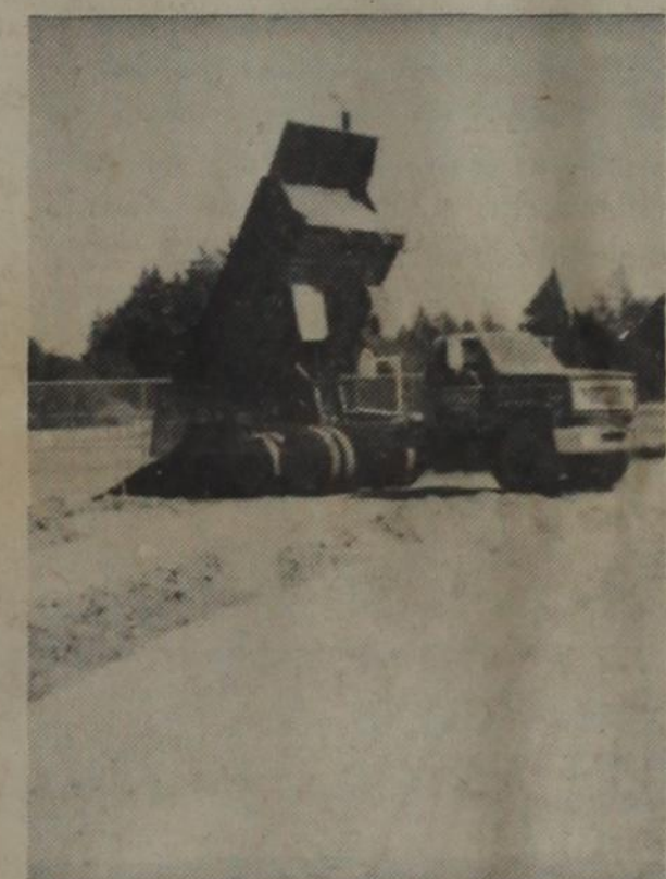
BUSY, BUSY — Work is still progressing on the New Cross Plains track. Here, dirt is being shifted by the tennis courts.
