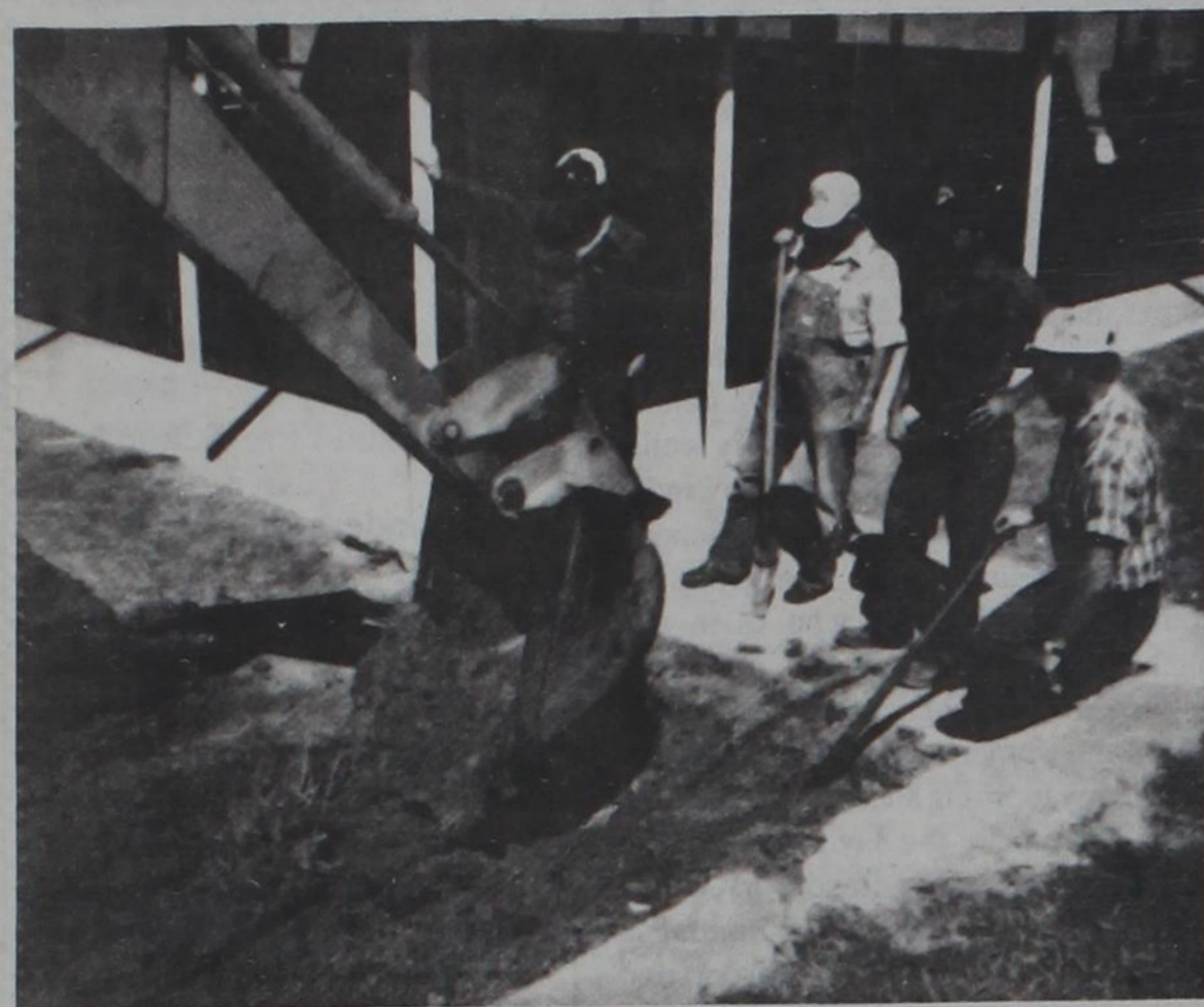
LOOKING FOR THE PROBLEM — Workmen are digging several holes on the high school grounds trying to find out why one of the sewer lines ruptured at school on Friday, September 24.
