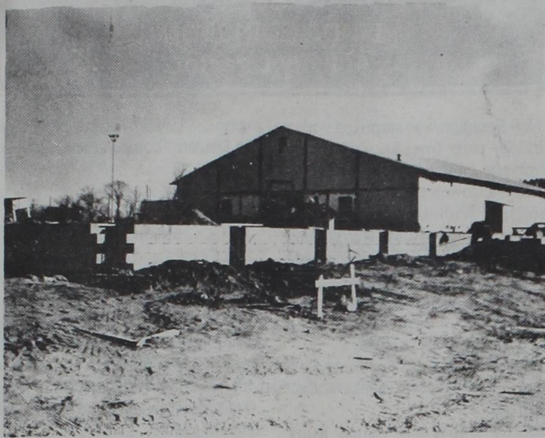
New Cross Plains High School Gym Construction Progressing — The new facility is located just west of the Buffalo Dome (the old gym) and is expected to be complete for next year's basketball season.
