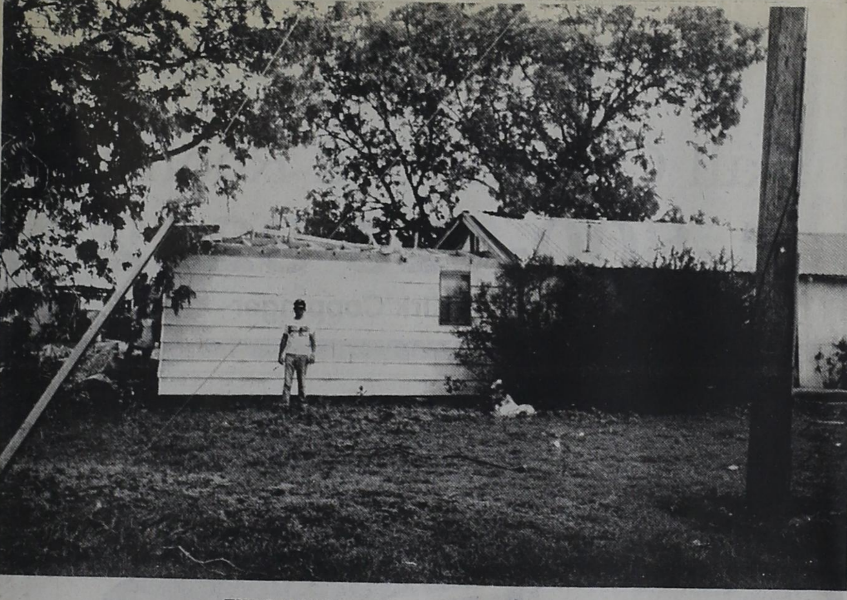
THE RAY WORLEY HOUSE LOSES PART OF ROOF
