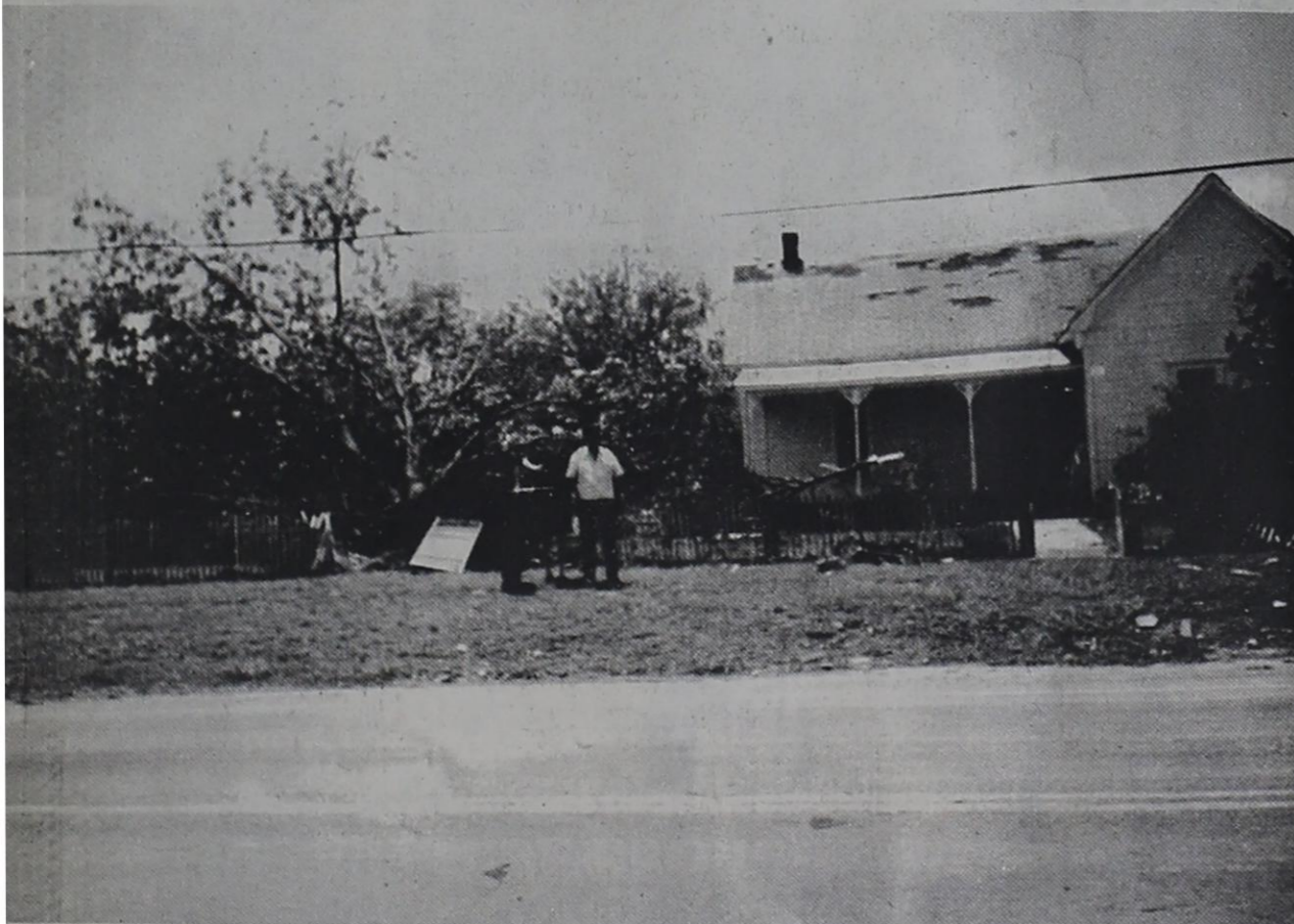
HOWARD HOUSE DAMAGED — picket fence and special gate are down, yard of the historic property, and a large tree was uprooted in the front
