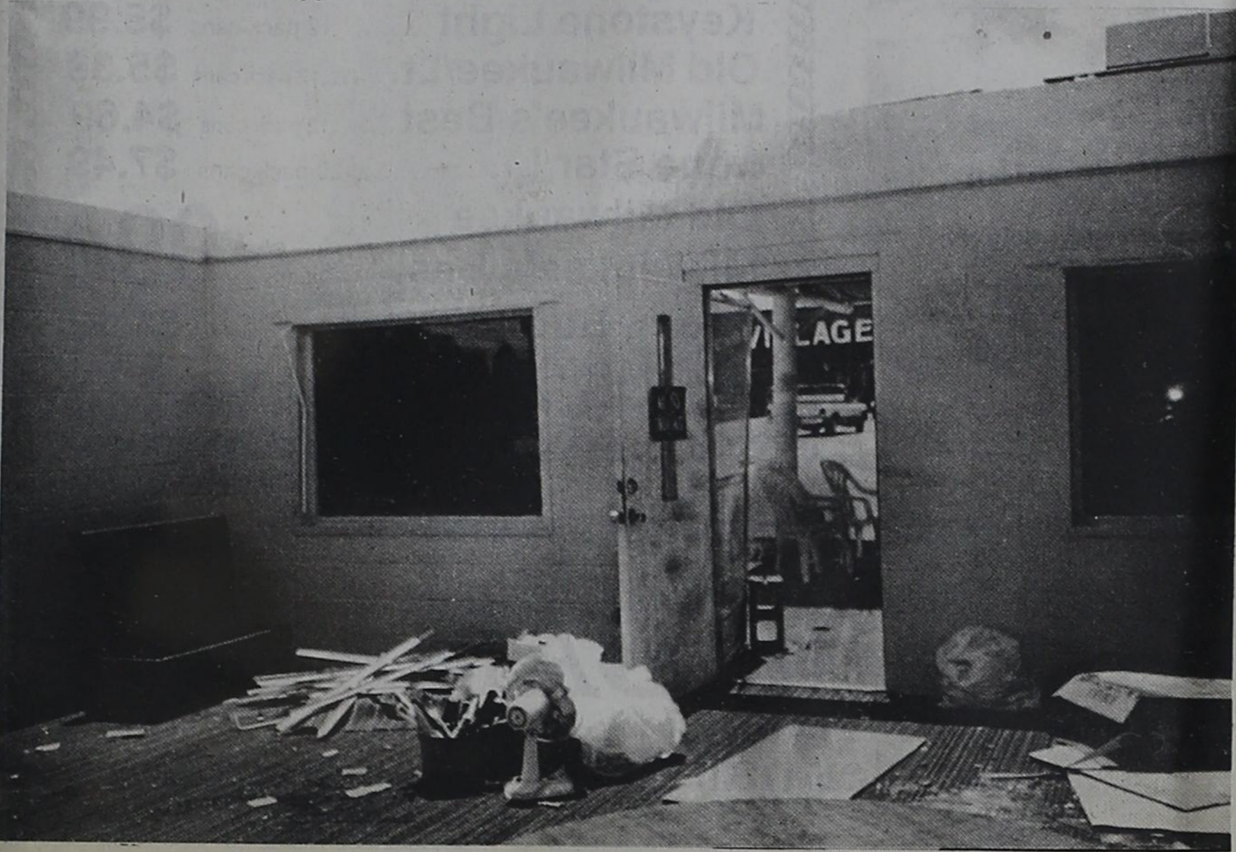
DINING ROOM AT JACK'S PLACE HAS NO SIGN OF A ROOF
