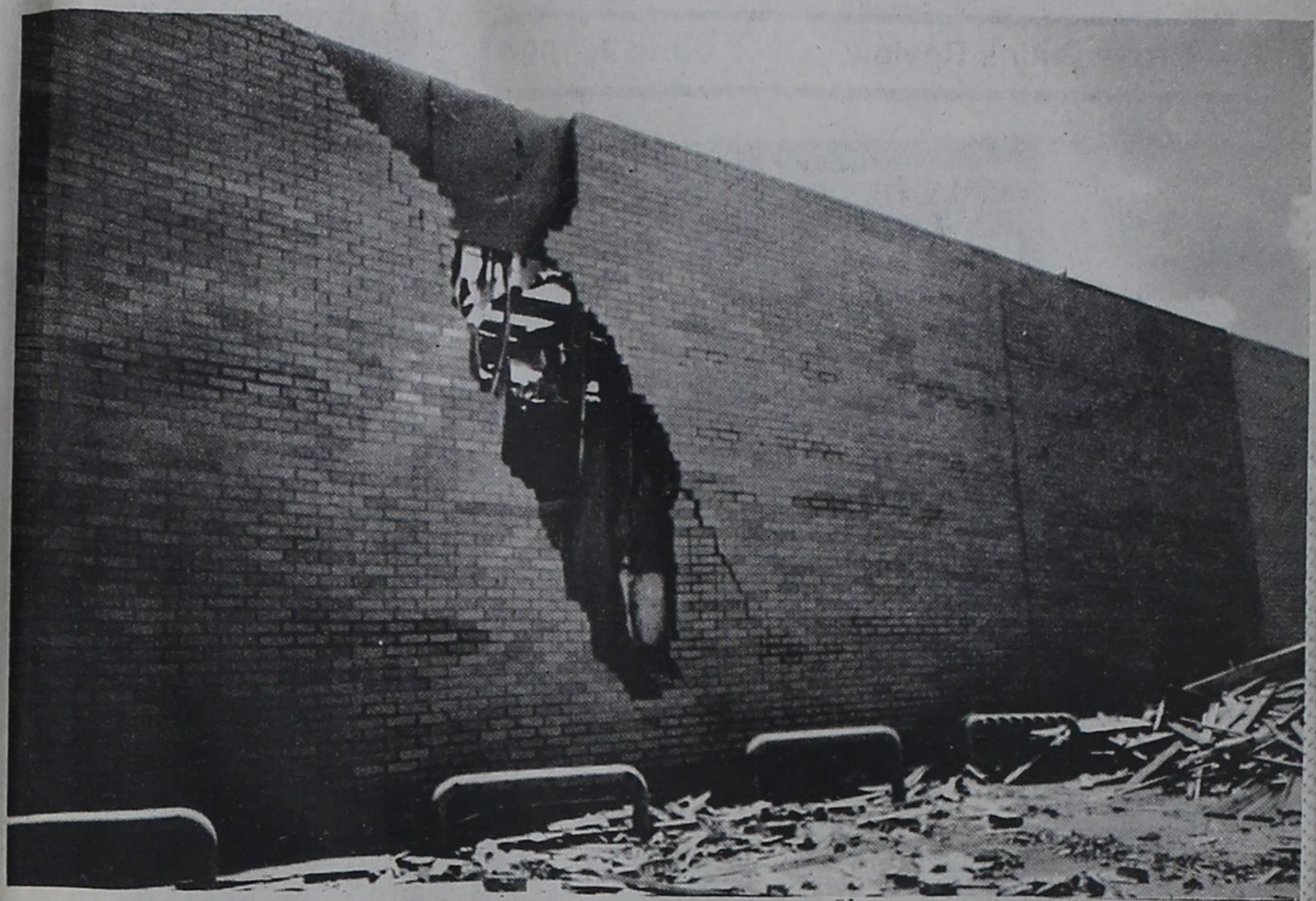
VILLAGE MARKET HAS GAPPING HOLE IN WEST WALL
