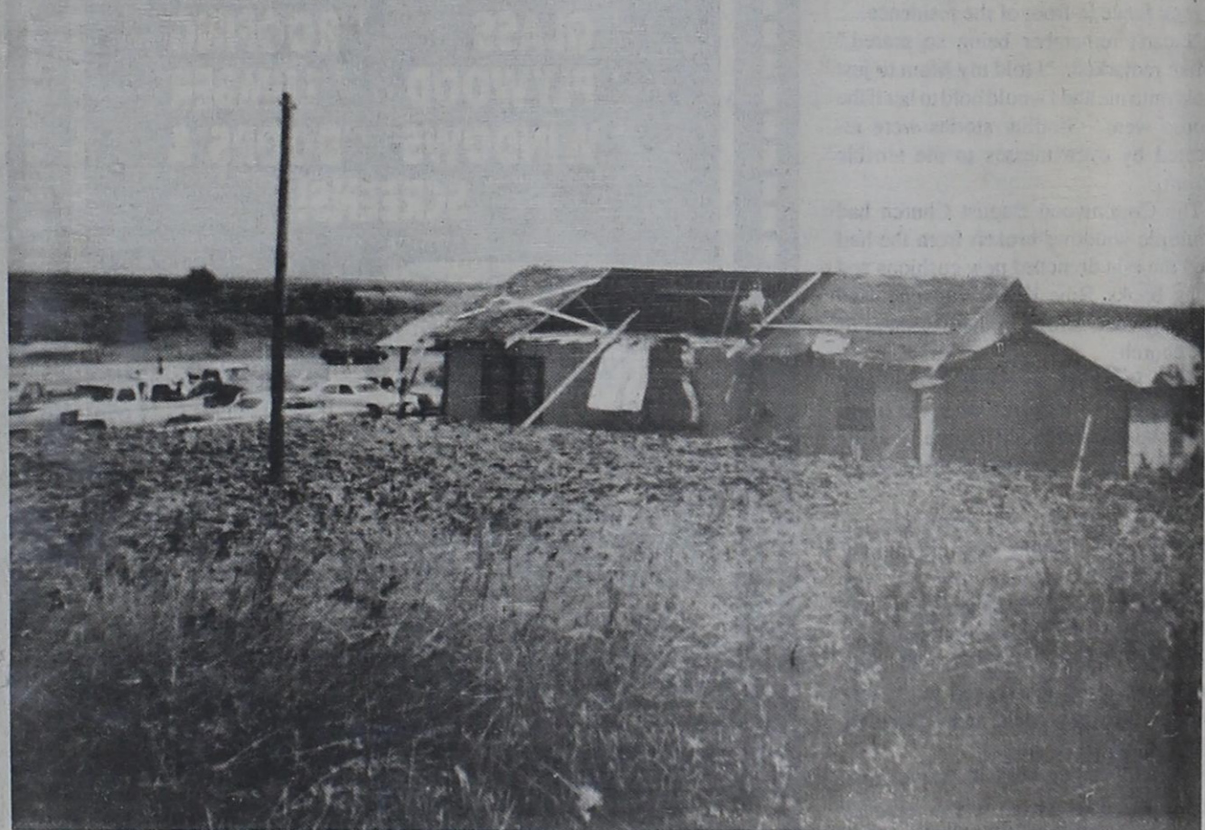
JAKE AND JULIE BYRD'S ROOF BEING REPAIRED FOLLOWING TORNADO WINDS AT CROSS CUT - CHIMNEY FELL ONTO HOUSE
