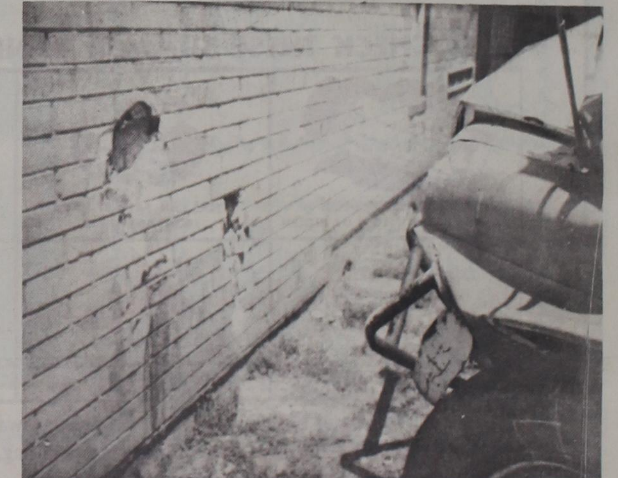
VAN LEAVES MARK ON SCHOOL BUILDING — The van which came unhooked left a couple of large indentures on the elementary building.
