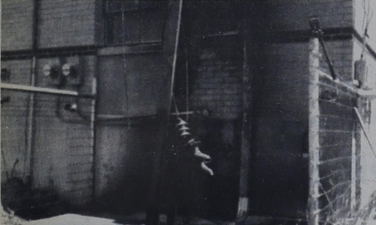
EARLY MORNING FIRE —Monday morning at 7:30 firemen answered a call at the city water filtering plant to find three transformers burned and the building damaged, the fire was already put out with fire extinguishers by City employees. Cause of fire is unknown, damage $3,500 transformers and some undetermined amount of damage to the building.
