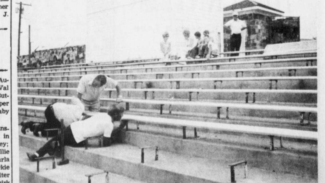
Volunteer workers are shown here bolting down the new aluminum bleacher seats at Broncho Stadium Tuesday afternoon. Watching from above at extreme left is Coach Noonkester's wife, Joan and at extreme right is high school principal Mark Gunnells. Staff Photo
