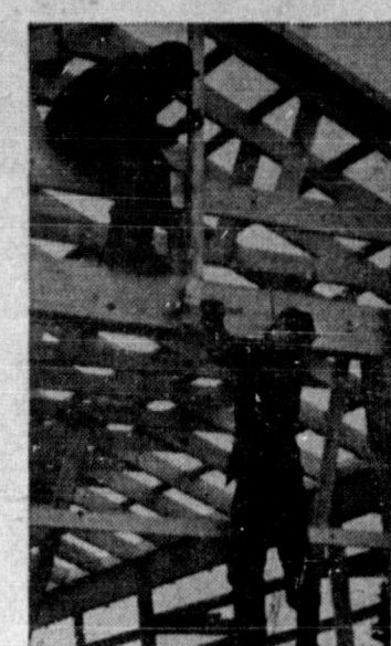
"ONE ARMY" Reserve Engineers of Anchorage, Alaska's Company B, 813th Engineer Construction Battalion ply their Army trade of constructing buildings at Ft. Richardson.
