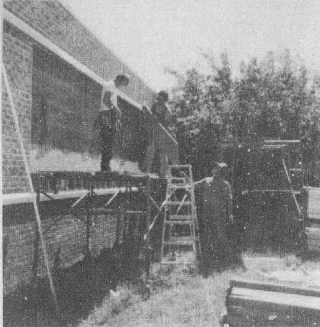
HIGH SCHOOL RENOVATIONS... The Renovations for the school began Friday, September 10. Plans have been made to lower ceilings, close windows and install heating and air conditioning. When completed, the high school will have a whole new look.
