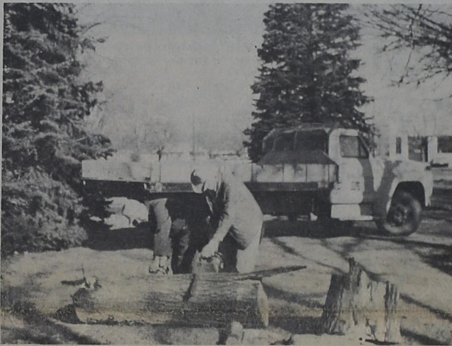
SATURDAY SEVERAL old dead trees were cut down and removed from around the courthouse. Working to clear the trees were Dale McGaugh, his son-in-law Buck Wehrlein of Canyon and Pete Land. In the future county officials have indicated they hope to replace the dead Chinese elm trees with a better variety of trees.
