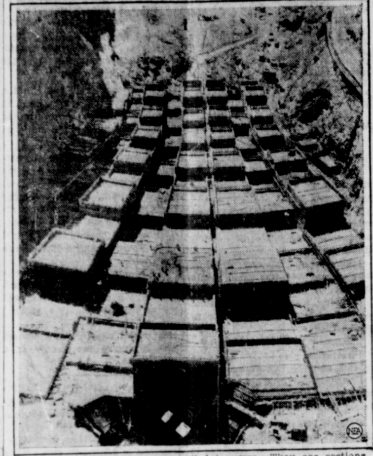
No, these aren't berry boxes piled in rows. They are sections of the foundations for Boulder Dam, the government's $165,000,000 hydroelectric project on the Colorado river. The size of the foundation works, which are built of concrete and steel, may be gauged by the small figures of men working on their surfaces.
