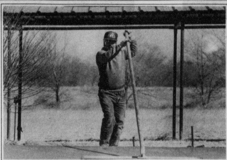
Jimmy Vela of Vela Concrete in Clovis smooths freshly poured cement. It is part of a new dance floor for the Immaculate Conception Catholic Church's annual Jamaica Festival in July.
