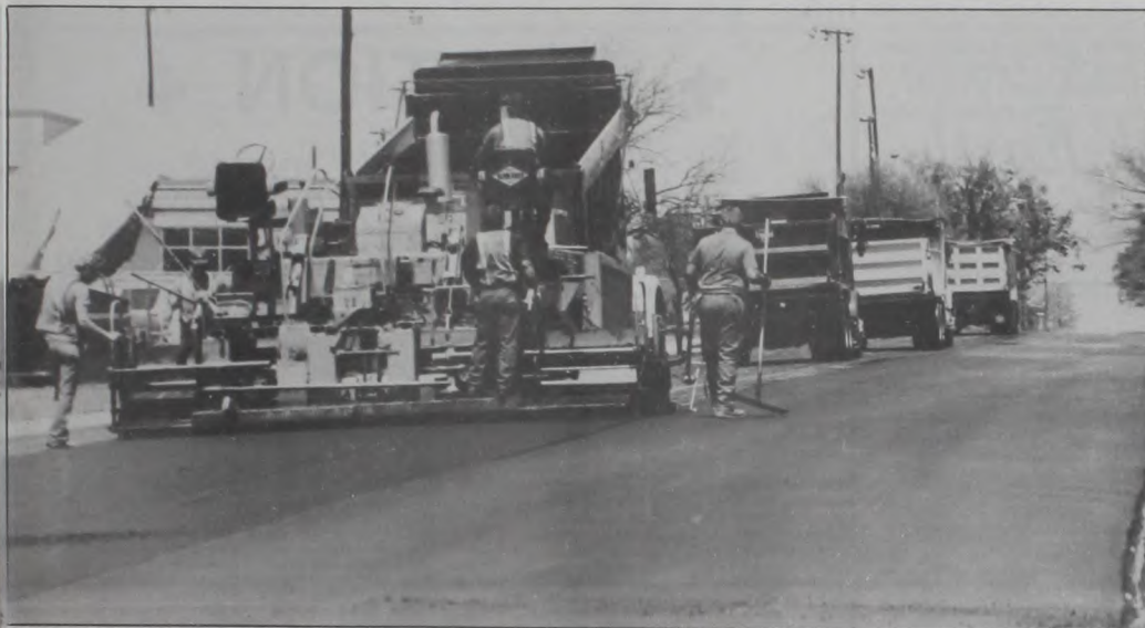
PAVING CREWS and equipment from Overland Corporation put new hot mix surfaces on N. Walnut and N. Hickory streets this week, just in time for Germanfest.
