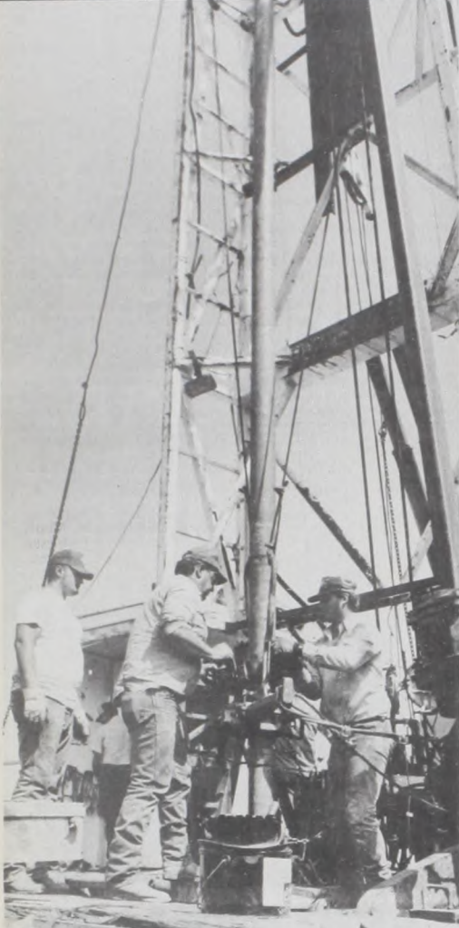
MUESTER'S NEWEST CITY WATER WELL is drilled by the crew of J.J. Biffle Water Well Company. Janie Hartman Photo
