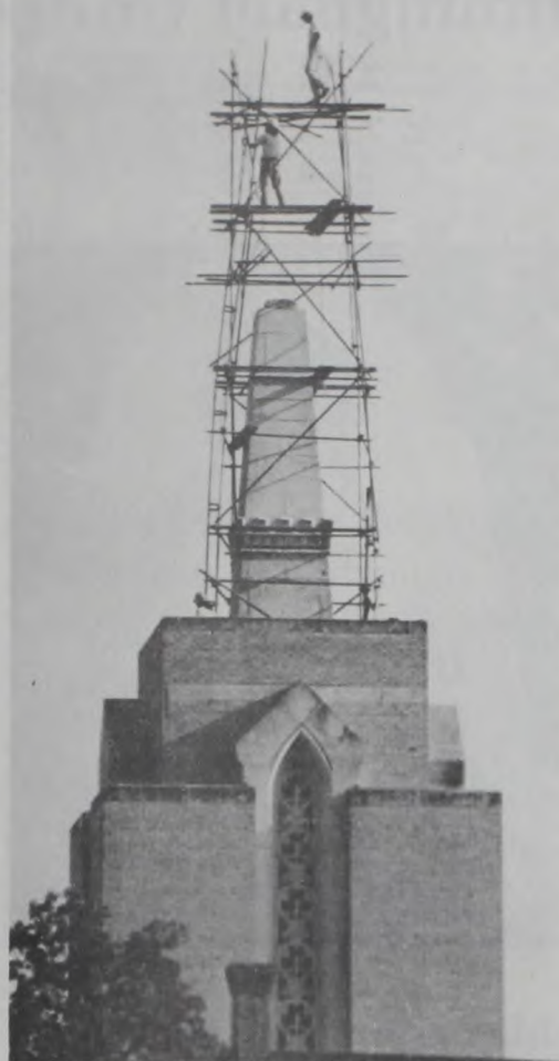
On top of the world. Workers remove a partial section of the scaffolds, then leave the fenced in steeple until plans for repairs are complete. Photo by Janie Hartman
