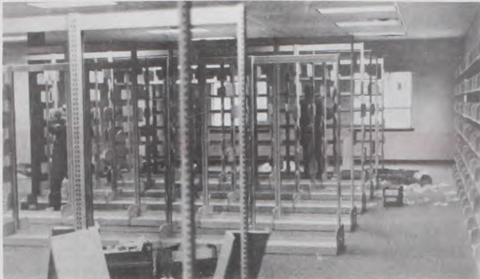
It was a busy week at the new Muenster Public Library as workers installed new shelving in preparation of moving into the building. Work at the new library was on hold, waiting for a grant from the Tocker Foundation to pay for new shelving and furniture. With the shelving in, the next step will be the moving of all the books and other items from the "old" library. This task will be the Eagle Scout project of Mitch Felderhoff and take place April 6,7,8. The library may need to be closed some of the following week for final preparations. The new library should be opened for business on Tuesday, April 17. Photo by Janie Hartman
