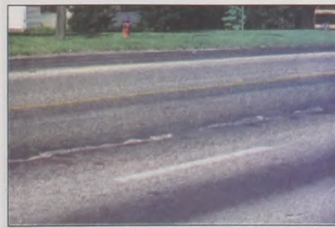
Road improvements?? TxDOT is working to correct problems with new seal coat. Janet Felderhoff photo
