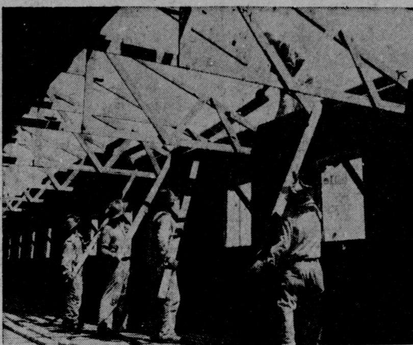
TWENTY-FOUR MILLION BOARD FEET of lumber are expected to be salvaged in the nation's first army camp demolition job now being conducted by War Assets Administration at Camp Hoenig, near Hoenig, Texas. Workmen are shown removing roof sheathing by the "strong-arm" method. Recovered building materials will be sold to priority holders for veteran housing.
