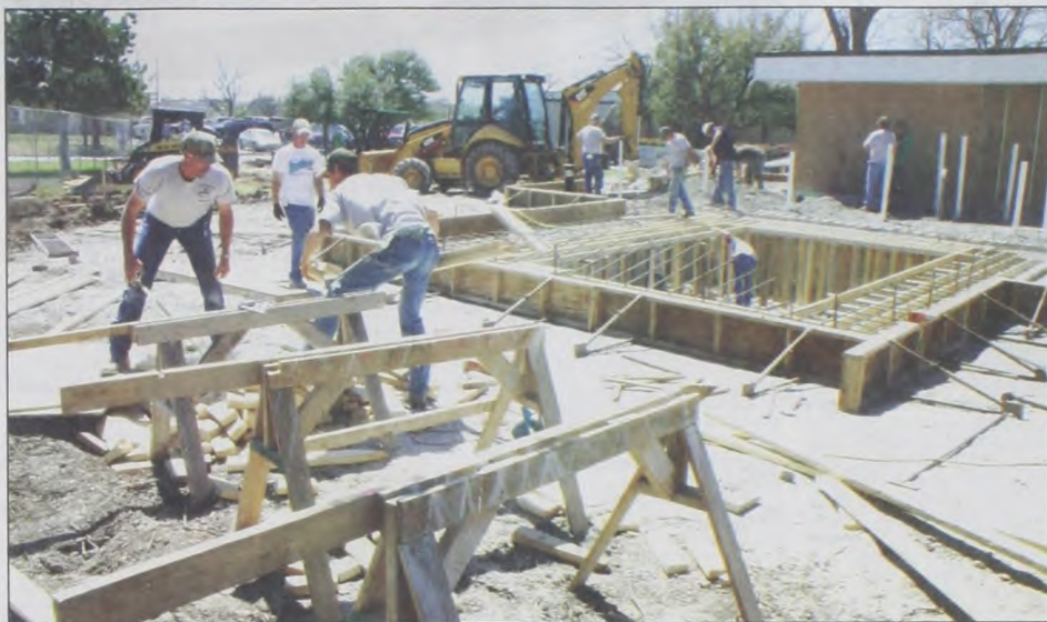
Progress continues to move swiftly along on construction of the new addition at Muenster Memorial Hospital. Presently, Dangelmayr Construction, Inc. workers are preparing to pour concrete for the hydrotherapy pool. When finished, the Hospital will have a very
