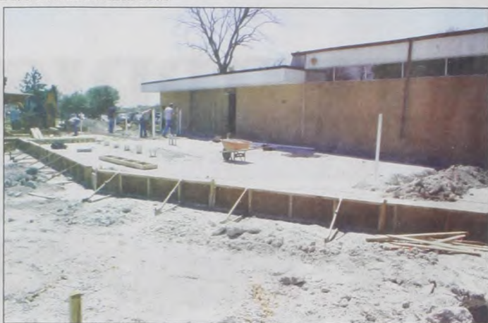
Muenster Memorial Hospital is in the process of getting a new front. Dangelmayr Construction, Inc. has been on the job all week doing prep work and pouring concrete for the new addition and front for the facility which is expected to be completed later this summer. Janie Hartman photo
