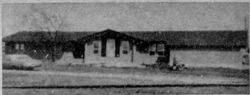
New home of Mr. and Mrs. Ray Wilde nearing completion in the northwest part of Muenster.
