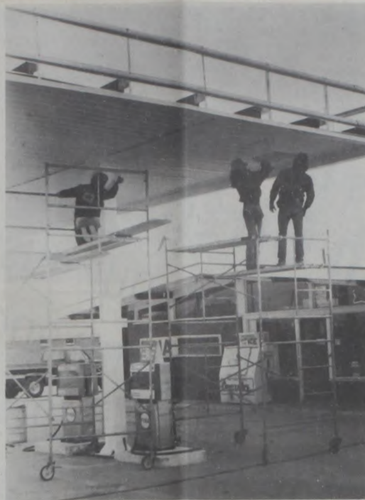
EMPLOYEES OF Charles Short Builders of Mabank, Texas are installing one of ten boxes for lights that will illuminate the ceiling of a new canopy at Schilling's Fina Station this week. When completed, Fina will paint in the Company colors of red, white and blue.
