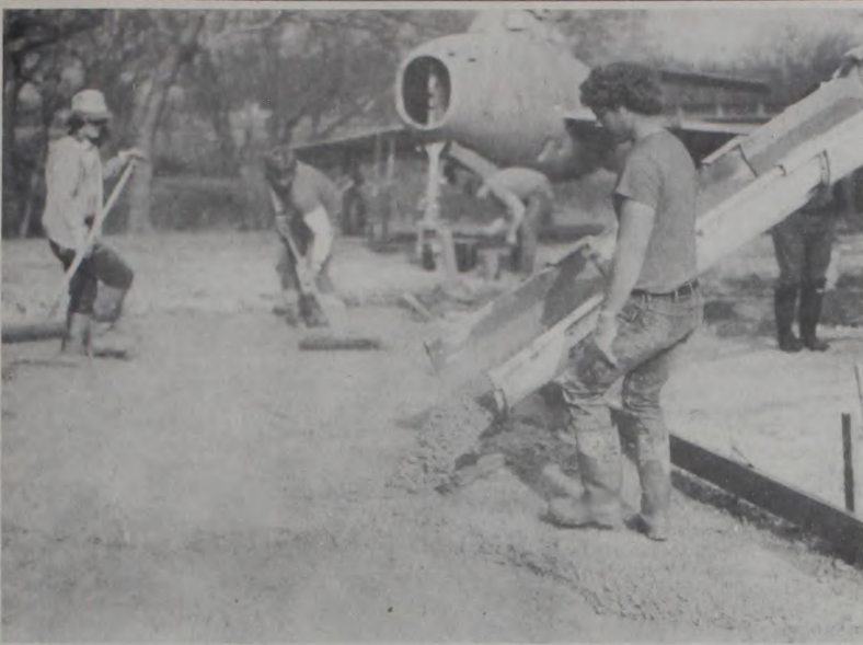
PHIL WALTERSCHEID directs the flow of concrete for a new section of roadway in the City Park Tuesday. The 30-foot-wide by 70-foot-long section is being funded by the Chamber of Commerce and will double as a dance floor for Germanfest. It will also serve as a demonstration job for possible concrete
