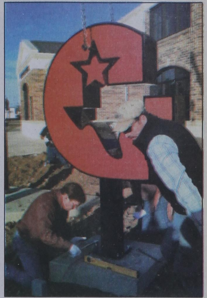
David Grotegut and Mike Yanke install a Gambler G in front of the new high school entrance. David made the Gambler G, and Ag Partners donated all materials, labor and paid for the paint job. Thanks Ag Partners for all you do for the school!
