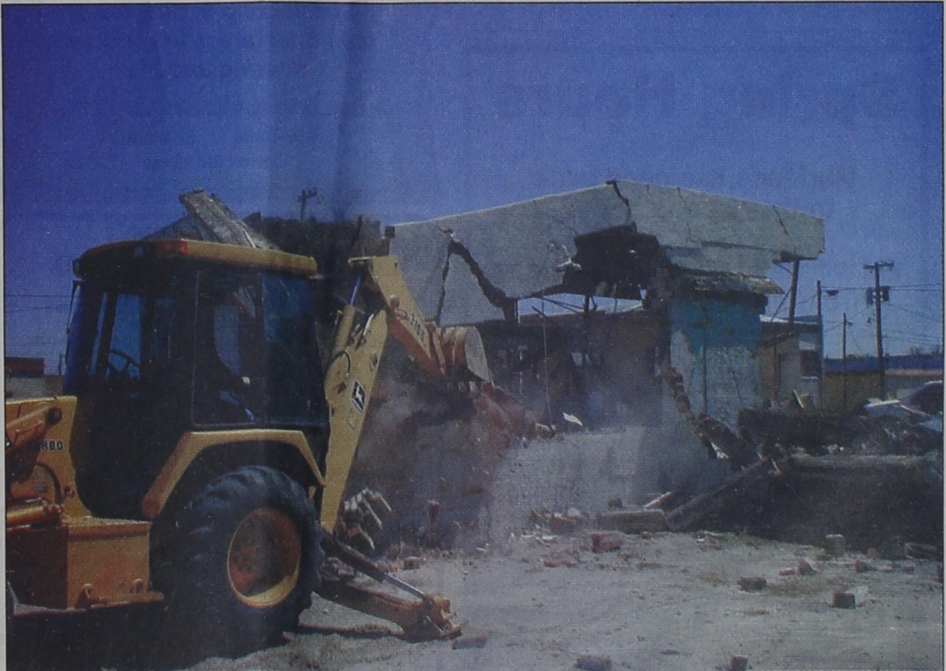
And the walls came tumbling down on a deserted building on Highway 15 in Spearman as Daniel Boyd and his front-end loader take a bite of brick.
