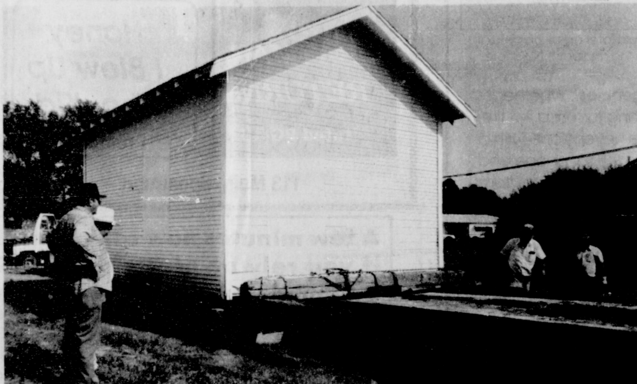
J.D. Wilbanks, Station Master's House Museum board member, and Don Reed, Transpecto, look on as Clarence Mitchell and Ron Dunnaway move to settle the little school house on its new foundation. The building was moved to the museum's lot on Thursday, Aug. 20. The house originally stood out by Horse Creek and is one of the oldest school buildings in the county. The house was moved by funds raised by the Twentieth Century Club.
