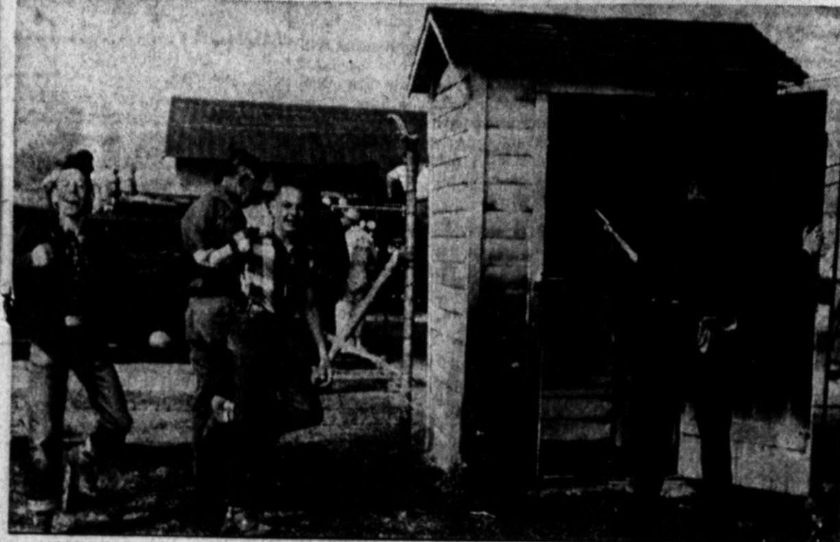
TICKET SELLERS for next fall's football games may not have to work in this building, which was damaged Thursday by a fire. The fire may have started from grass which was being burned off along the fence. Eighth grade football players, two of whom are shown at left, received the credit for discovering the fire. Kenny Wilson, right, was one of the first volunteer firemen at the blaze. (Staff Photo)
