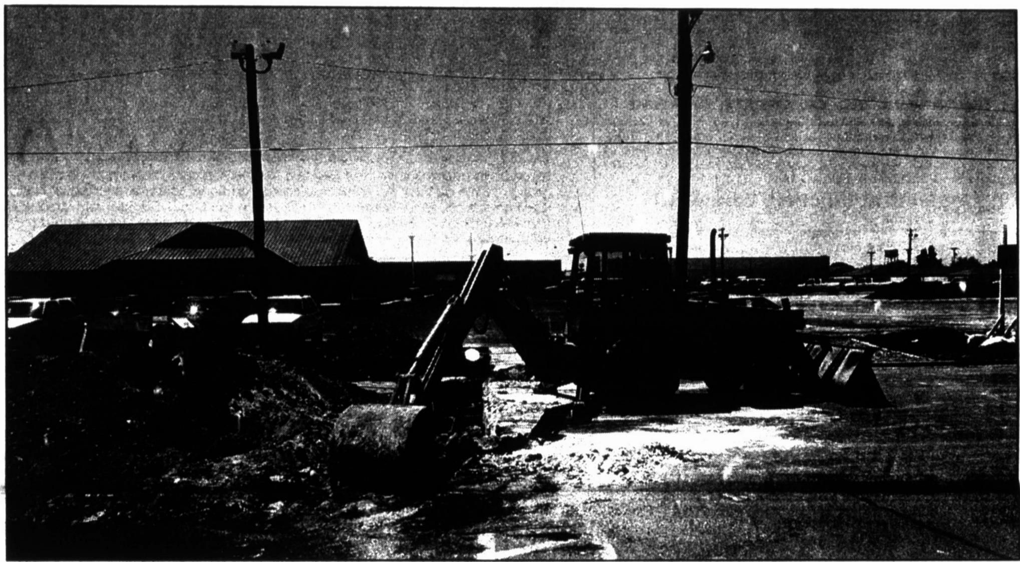
New sewer line — City of Hereford workers have been removing an old sewer line that crosses 15th Street between the Hereford Independent School District Administration Building and Stevens 5-Star Car & Truck Center. The line had become corroded, requiring replacement.
