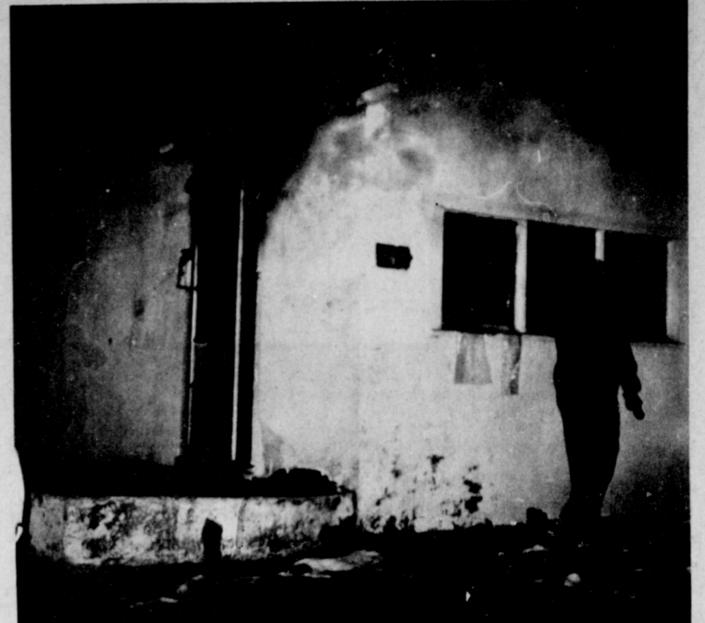
FIRE DAMAGES HOME. The Mentie Lewis Home at 911 West Avenue E received heavy damage Thursday night in a fire which broke out in a bedroom area. Fire officials suspect the fire originated in the attic, spreading in the attic. Heaviest damage was confined to a bedroom, although all of the house received damage in varying degrees.
