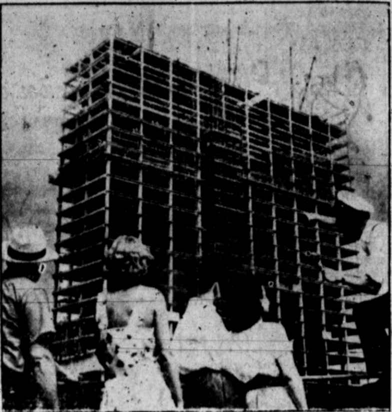
FRAMEWORK OF PEACE-Onlookers gaze at the progress being made on the new United Nations location in New York City. In the background is the skeleton of the U. N. Secretariat building, the first and tallest on the site. This 29-story structure will have 2700 air-conditioned offices.
