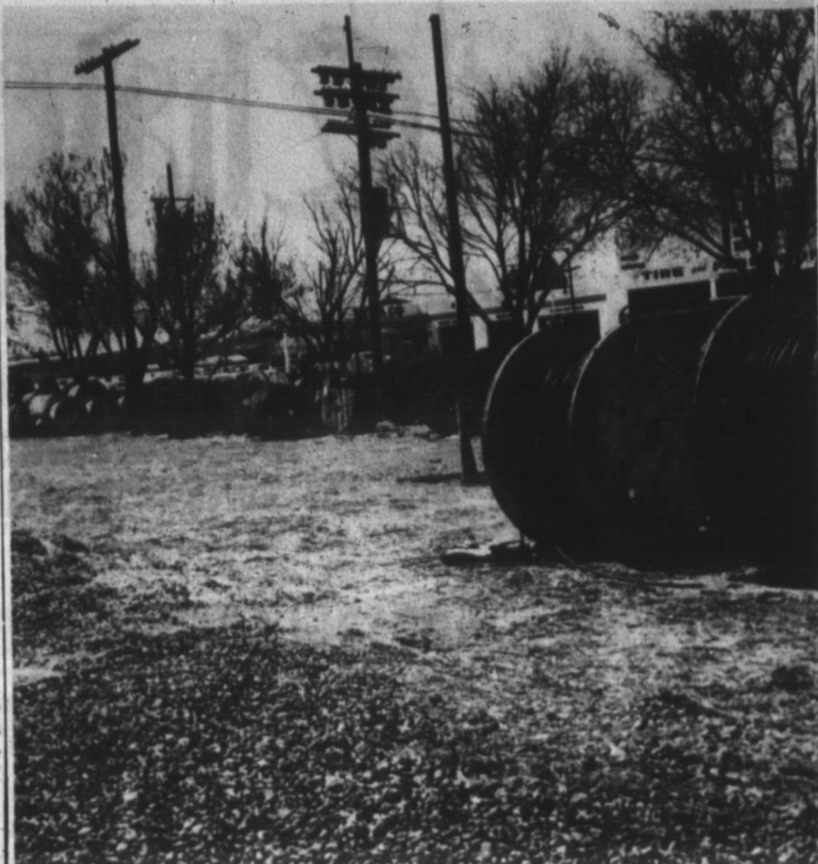
MILES OF WIRE — West Texas Rural Telephone Co. is going underground, literally. In an elaborate revamping of its telephone service, the co-operative is burying its main cables to provide better interstation service for its customers. This shows a small part of the underground cable stored on Santa Fe lots, ready for use by the cooperative as it broadens its service. (Brand Staff Photo)
