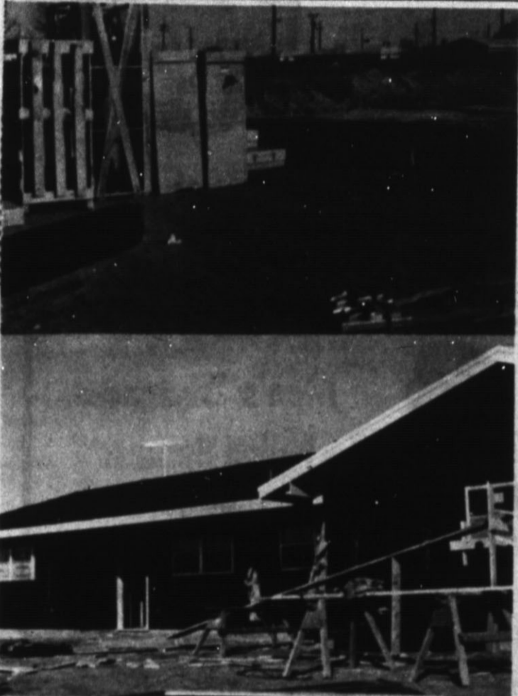
SOUTH STATES OIL CO. has a new business under construction on the corner of North 25 Mile Avenue and Vogle St. Bottom photo is a house under construction in Hereford's north residential area. —Staff Photos
