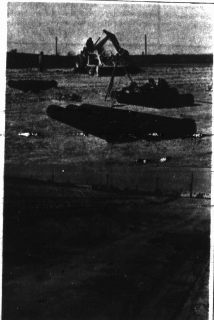
STILL PROGRESSING — Work at the Wilson and Company packing plant is still progressing as in the top photo workmen are digging trenches for the laying of pipe and in the bottom photo, they are preparing foundations for the pouring of concrete at the base of the building.
