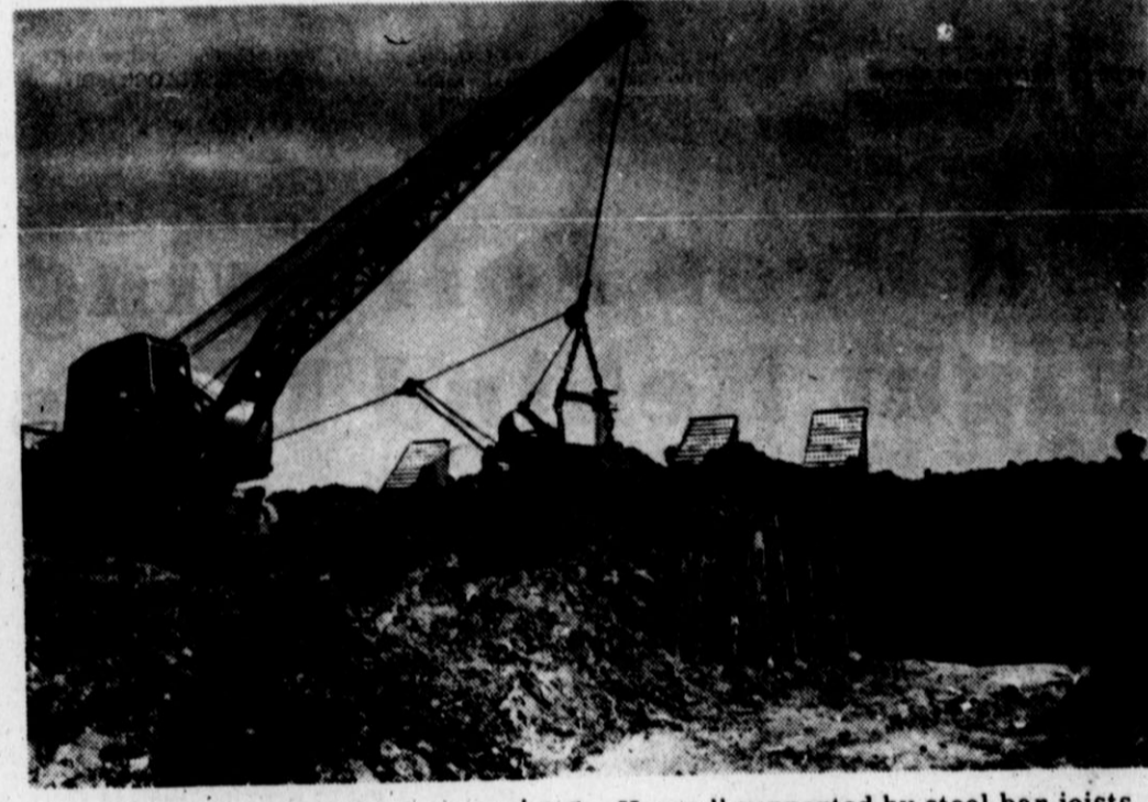
COVER-UP - Earth-moving equipment works during completion of an experimental home in Longmont, Colo. One foot of earth covers roof of this "Sun Earth Home," supported by steel bar joists and concrete deck. The earth slopes gently to the ground around most of the building. Several skylights and glazed windows provide light to the rooms.
