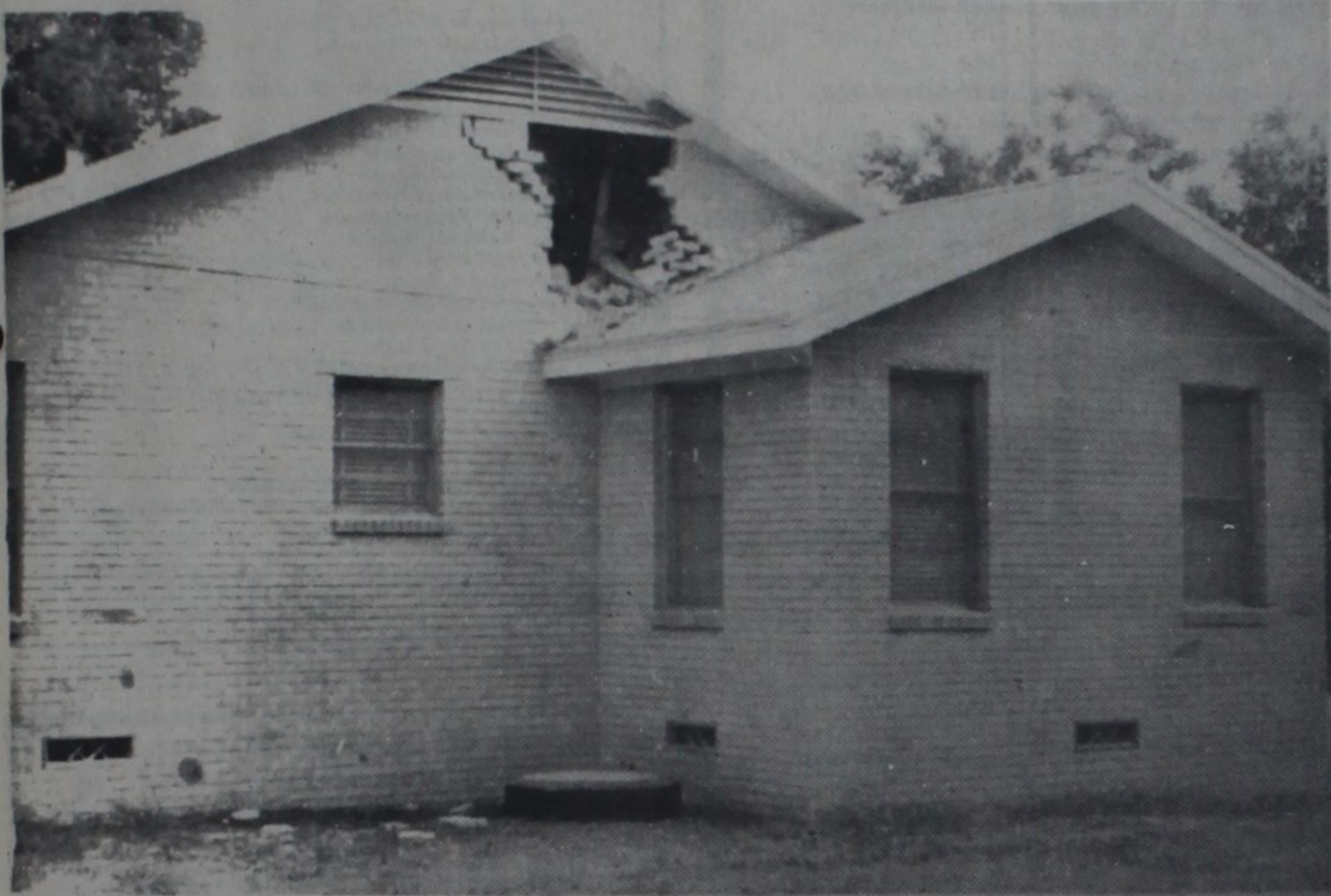
The home of Mrs. D. Breeding was damaged in a freak accident July 29.
